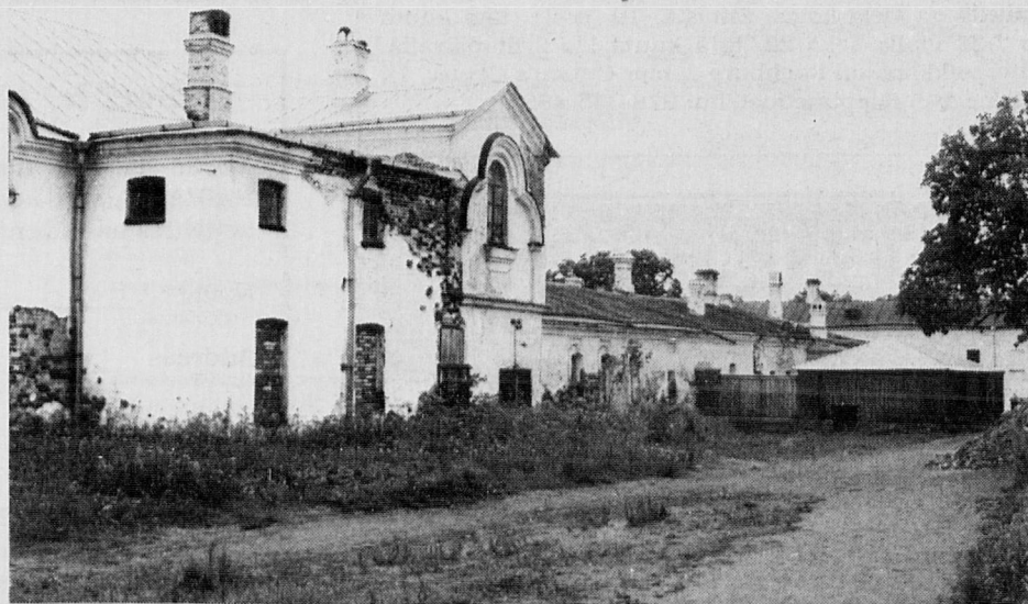
Vanha Valamo Monastery, showing the extent of disrepair.
