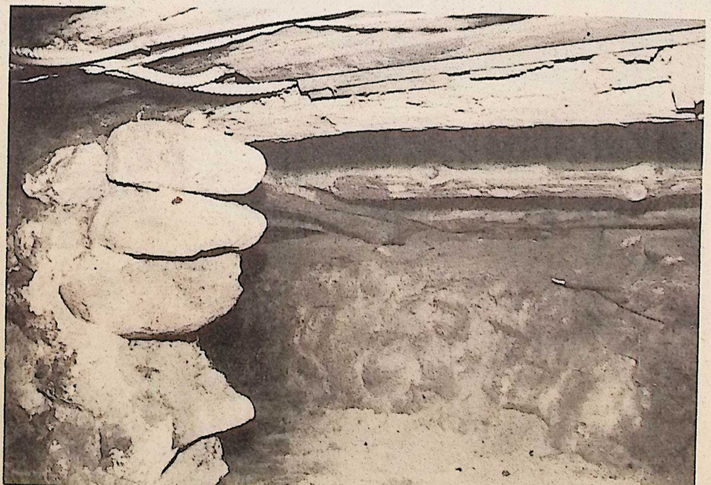
Photo shows the hand-hewn tree trunks which comprise the floor joists for the
